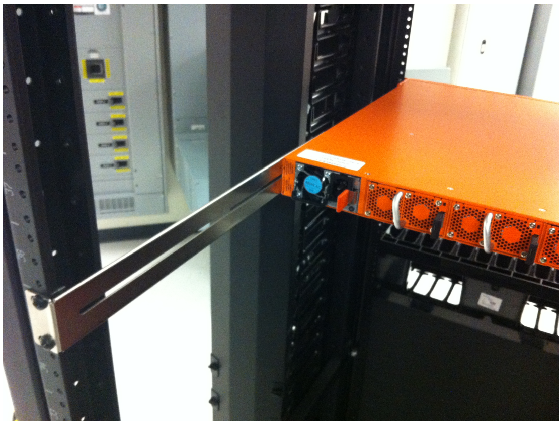
Figure 6 Rear View of the Mounted Node and Rails on the Four-Post Rack
